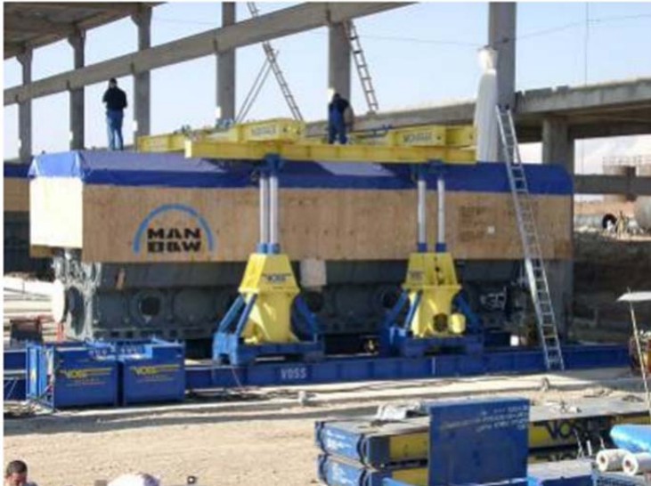
Unloading and transport of 4 Diesel engines each 270 tons to the foundation of the power plant in Batman, Turkey.
